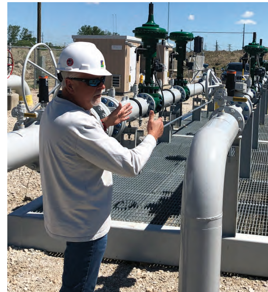
Photo courtesy of North Coast Gas Transmission
