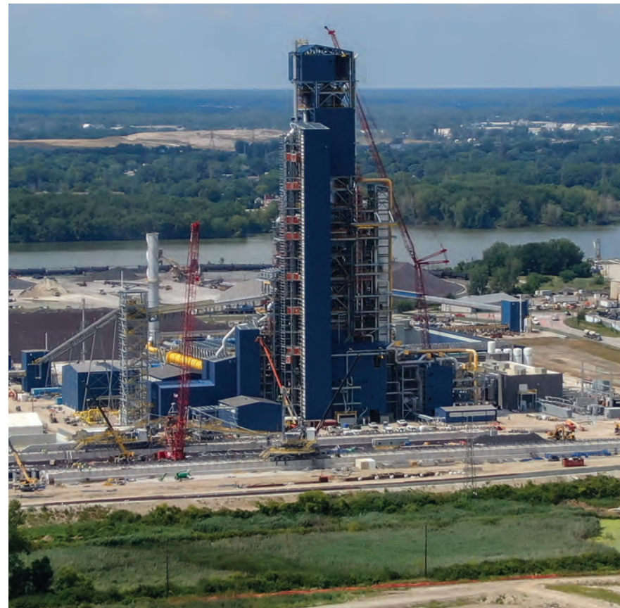
Cleveland-Cliffs’ new $700 million HBI facility in Toledo has capitalized on the region’s abundance of natural gas through the North Coast Gas Transmission pipeline. Photo courtesy of RGP
